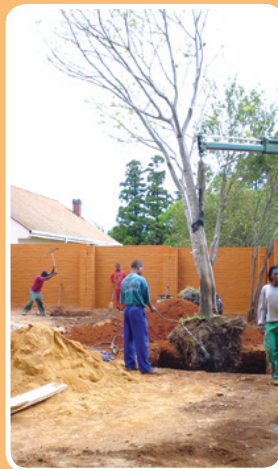
TOP: Back of Orejen prior to renovation. MIDDLE: Back of Orejen after renovation. BOTTOM: Replacement trees being delivered.
